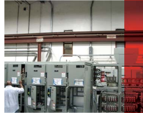
Drive & MCC String Testing
